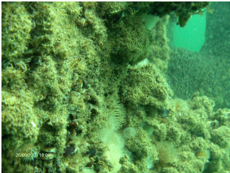
Picture 3: Marine growth on the monopile
